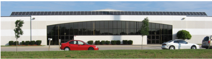
The 55 solar panels mounted on the roof of the Bethany Community Church generate revenue and support for renewable energy in the Niagara Peninsula.
